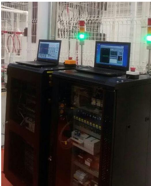
HCTS Control Cabinet + AC Apply Voltage Control Cabinet with
