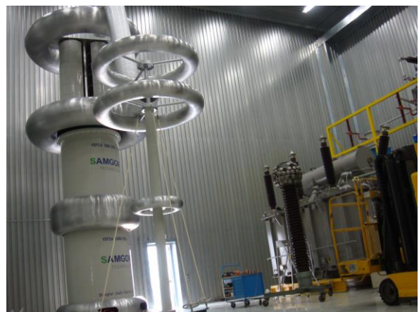
Shielding Room for 220kV Power Transformer
