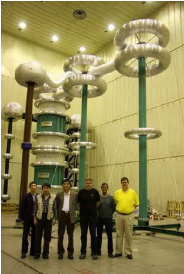
SGM3200KVA/800KV Helsinki University (Finland)
