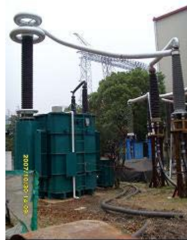
350KV/10A Tank type Tunable Reactor Resonant Test System
