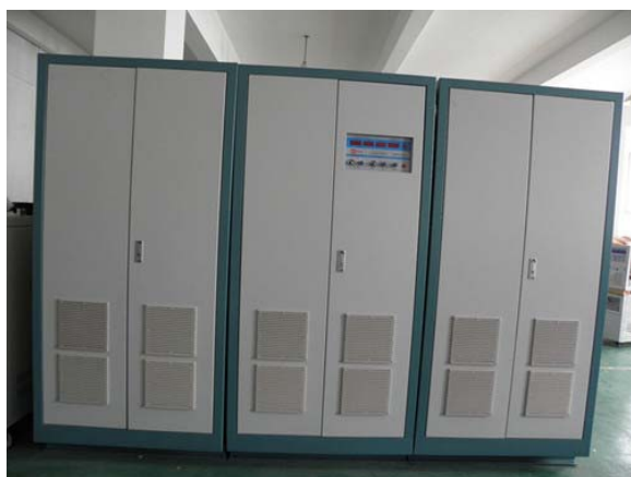
1000kVA PWM IGBT Power Source (3 phase)
