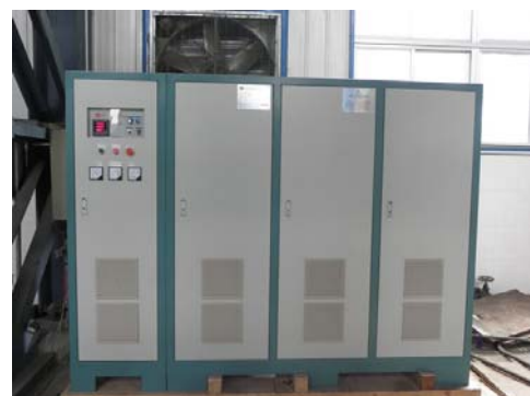
600kVA PWM IGBT Power Source (3 phase)
