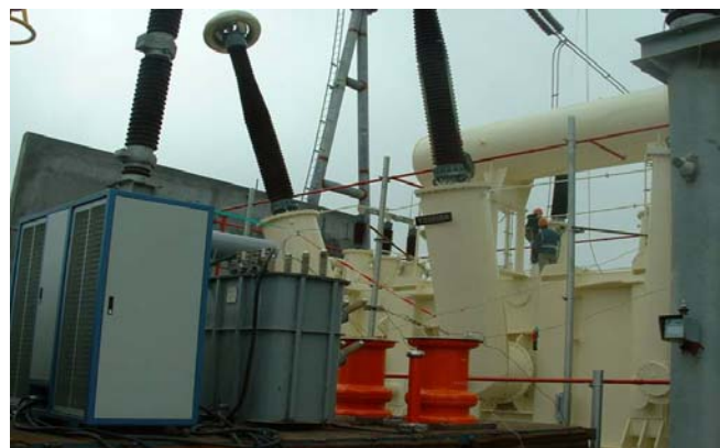
550kV Power Transformer Onsite Induce Voltage Test
