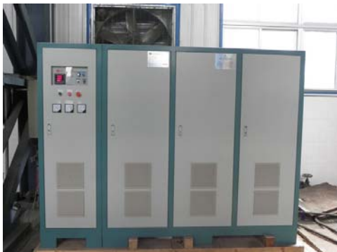
600kVA PWM IGBT Power Source (3 phase)
