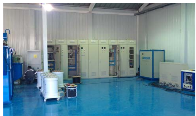
50kVA PWM IGBT Power Source (3 phase) for Induce Voltage Test
