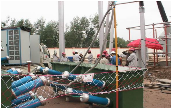
750kV Power Transformer Onsite Induce Voltage Test
